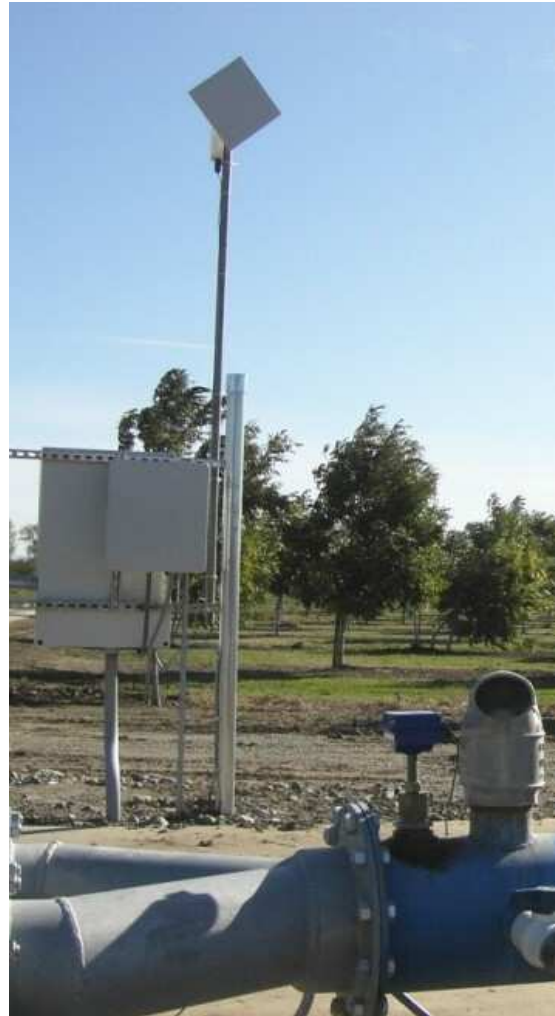
Figure 3, 5.8 Ghz Ethernet bridge end-point at pump site
